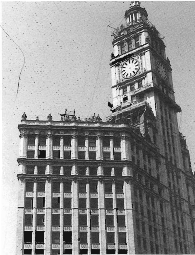
Work in progress on the Wrigley Building. The same natural forces that weather and weaken stone surfaces have attacked this structure's gleaming white cladding. Molded plastic replicas now replace the original terra-cotta tiles.
