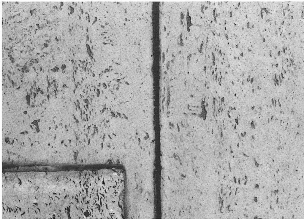
Travertine, an unusual carbonate rock, has been a favorite of architects for centuries. Here on the Seventeenth Church of Christ Scientist, the pockmarks characteristic of this stone form a linear texture that runs perpendicular to the ground.
